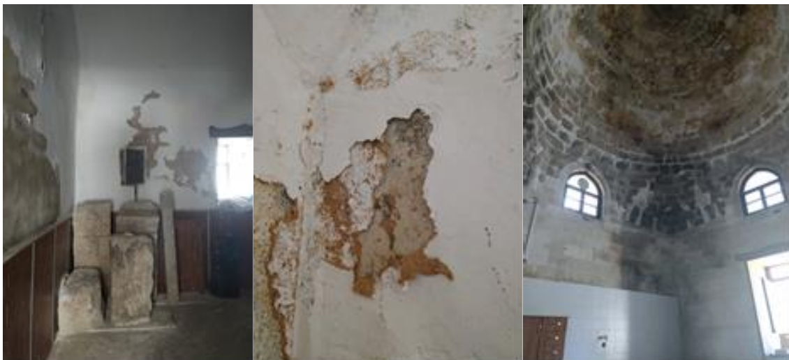
Figure 6. Material deterioration in different parts of Karaman Hatuniye Madrasa.
