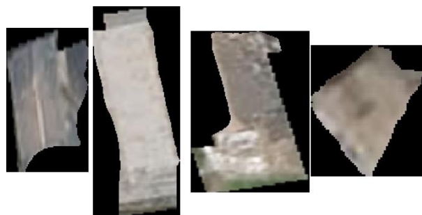
Figure 8. Examples of image of roof surf with damage (damage (-25 %), damage (25–50 %), damage (50–75 %), damage (75%) ordered from left to right)
