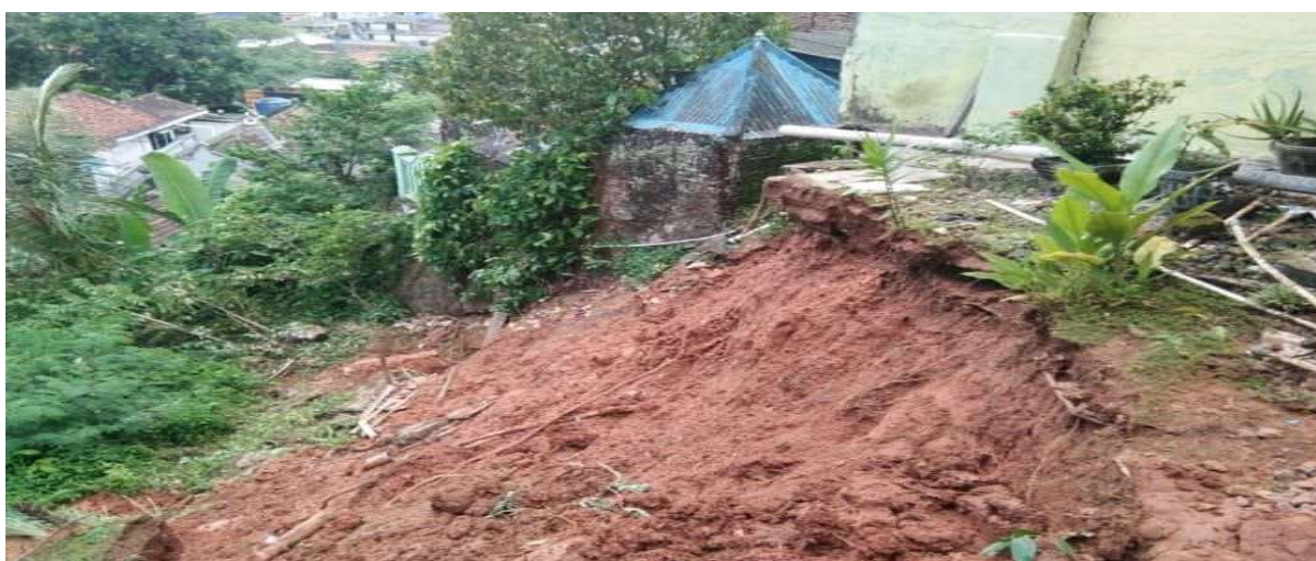
Figure 2. Houses affected by landslides due to heavy rains in Panjang sub-district (Kumparan, 2019)
