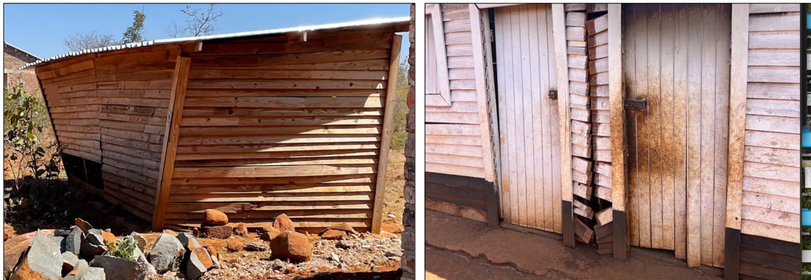
Figure 7. Damaged Phase 1 unit - West End (Ward 7) (Photography by Author, 2023)
