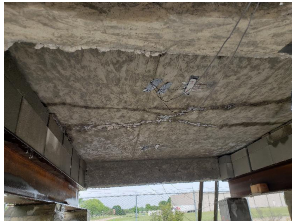
Figure 6. Observed cracking in slab
